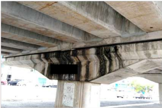
Figure 1 Bare concrete surfaces of a bridge with excessive dampness
